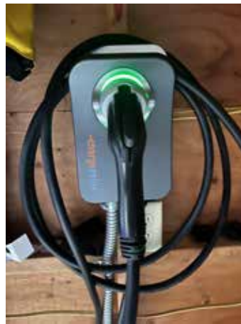
Level 2 Home Charging Station (you might get a tax credit for installing one of these)
